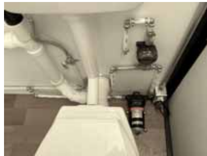
Water Pressure Pump With Filter and on and off switch.
